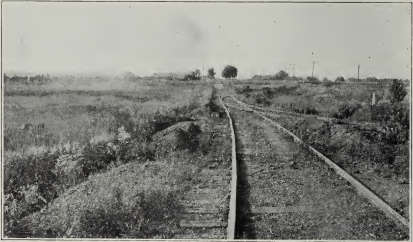
FIG. 38.—Railroad track in Franklin County lowered by surface subsidence resulting from room-and-pillar mining of a 9-foot coal at a depth of 425 feet. The maximum subsidence was 4 feet. The track has been partially repaired.
